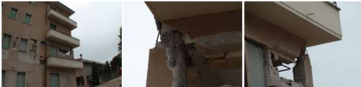
Figure 6. Joint failure due to infill damage – L'Aquila earthquake (photos by K. Mosalam)
