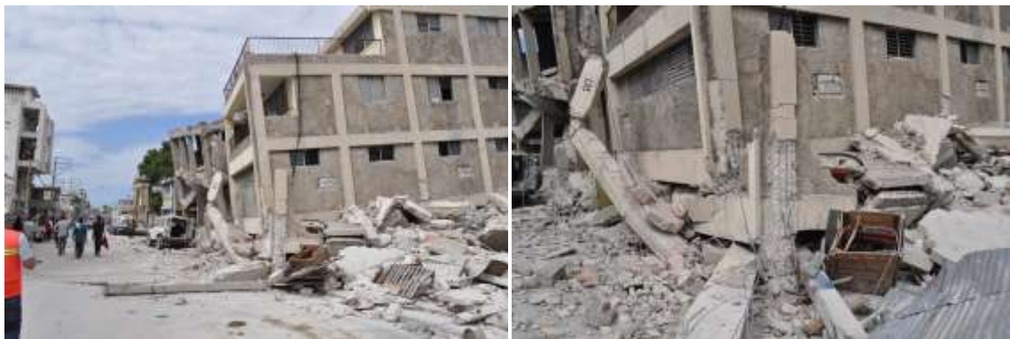
Figure 8. First story collapsed building – Haiti earthquake (photos by E. Fierro)
