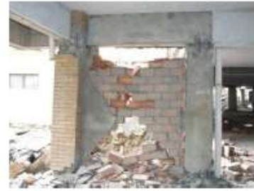
(f) Infill wall shear damage and major frame damage
