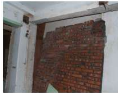
(b) URM infill wall damage and negligible RC frame damage
