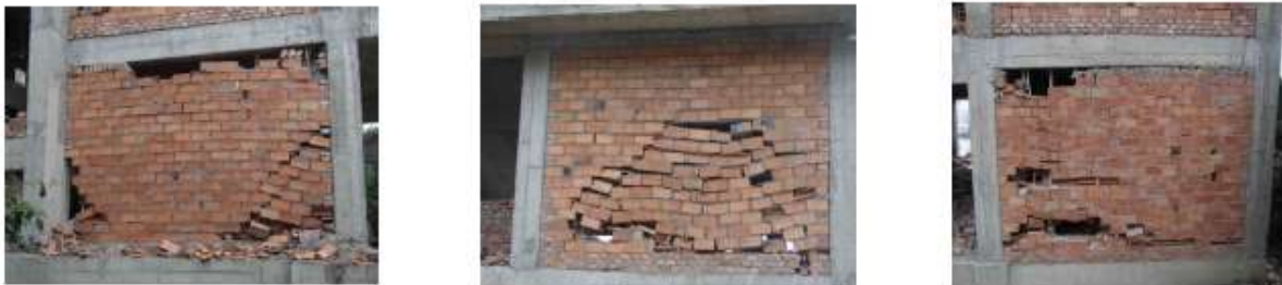
(a) Infill wall compression and shear damages
