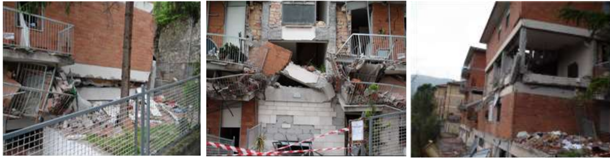
Figure 5. Story collapse due to infill failure – L'Aquila earthquake (photos by K. Mosalam)
