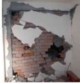
(e) Infill wall compression and shear damages and moderate frame damage
