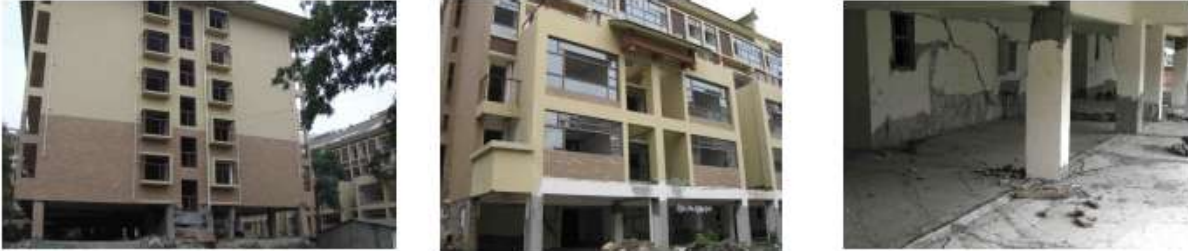
(a) Major damage
