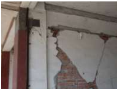
(a) Moderate damage to RC frame and URM infill wall
