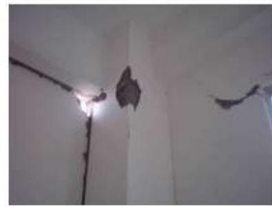
(c) URM infill wall damage and minor RC frame damage
